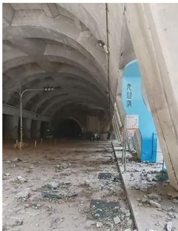
Figure 1-2 Open-cut tunnels with EPS foam cover after rockfall events.
