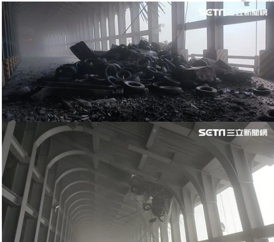
Figure 1-3 Open-cut tunnels with recycled tire cover collapsed after rockfall events. (SET News)
