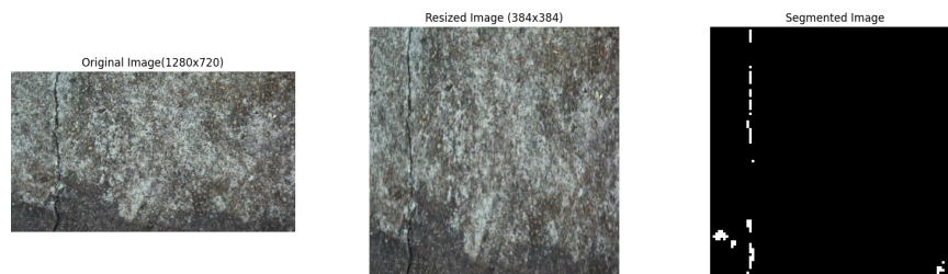
Figure 3.9: At point A, the segmentation results of the detected crack are obtained. After detecting the crack, the segmented image data is fed into DDQN (Double Deep Q-Network) for prediction, followed by forward flight.
