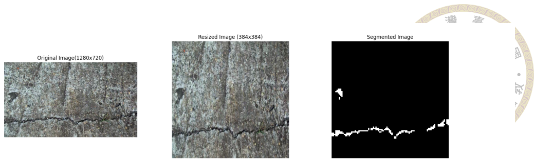
Figure 3.15: At point G, the segmentation results of the detected crack are obtained. After detecting the crack, the segmented image data is fed into DDQN (Double Deep Q-Network) for prediction, followed by a flight towards the right.
