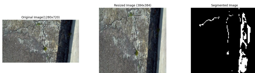
Figure 3.18: At point J, the segmentation results of the detected crack are obtained. This is the endpoint, so no further flight is necessary.
