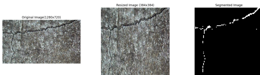
Figure 3.12: At point D, the segmentation results of the detected crack are obtained. After detecting the crack, the segmented image data is fed into DDQN (Double Deep Q-Network) for prediction, followed by a flight towards the front-right direction.
