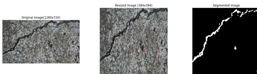
Figure 3.14: At point F, the segmentation results of the detected crack are obtained. After detecting the crack, the segmented image data is fed into DDQN (Double Deep Q-Network) for prediction, followed by a flight towards the front-right direction.
