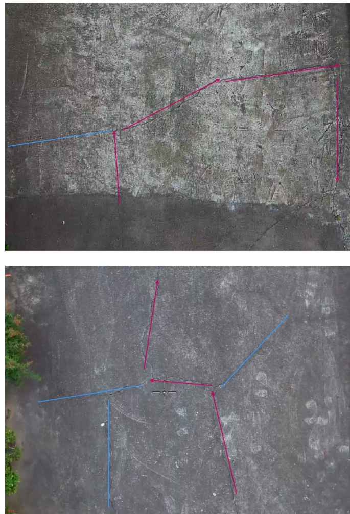
Figure 4.1: Test A and Test B environments, with red indicating the path where they capture cracks, and blue showing the missed area.
