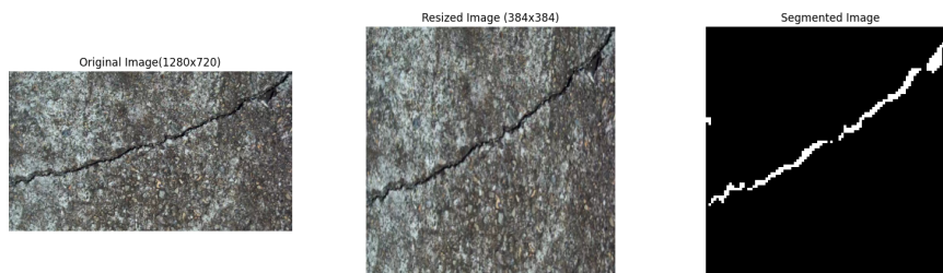
Figure 3.13: At point E, the segmentation results of the detected crack are obtained. After detecting the crack, the segmented image data is fed into DDQN (Double Deep Q-Network) for prediction, followed by a flight towards the front-right direction.
