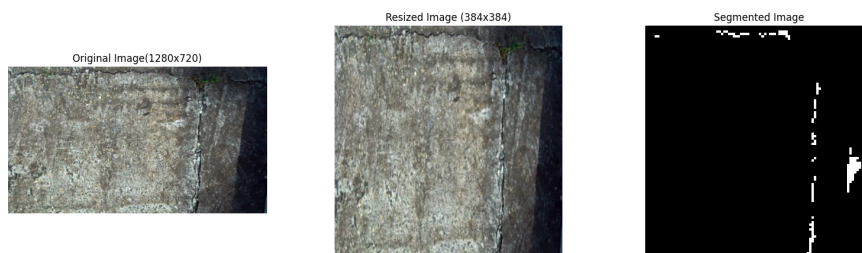
Figure 3.16: At point H, the segmentation results of the detected crack are obtained. After detecting the crack, the segmented image data is fed into DDQN (Double Deep Q-Network) for prediction, followed by a flight towards the back.
