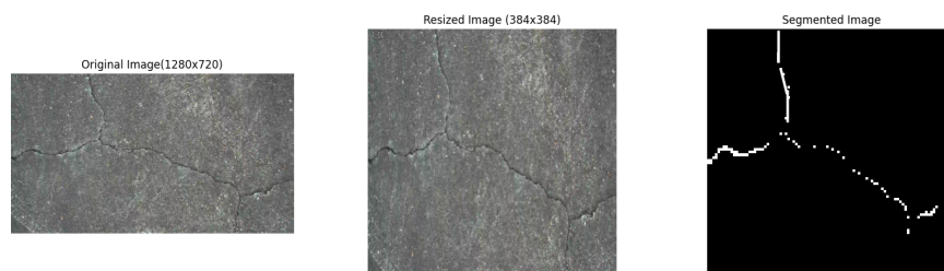
Figure 3.24: At point d , upon obtaining the crack segmentation results, the drone determines forward flight direction using DDQN.
