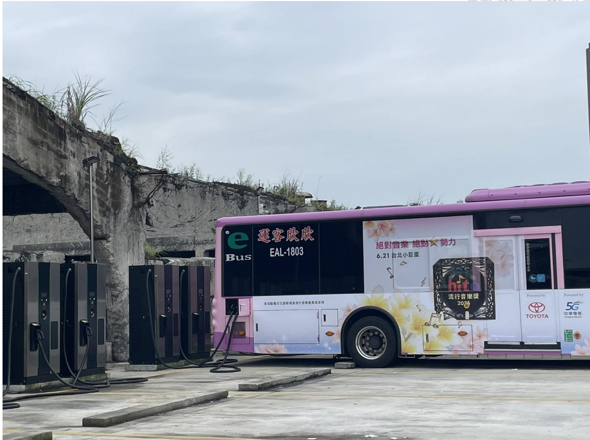
Figure 59 Charging Allocation with Electric Buses in Xinxin Bus Zhongxing Depot
