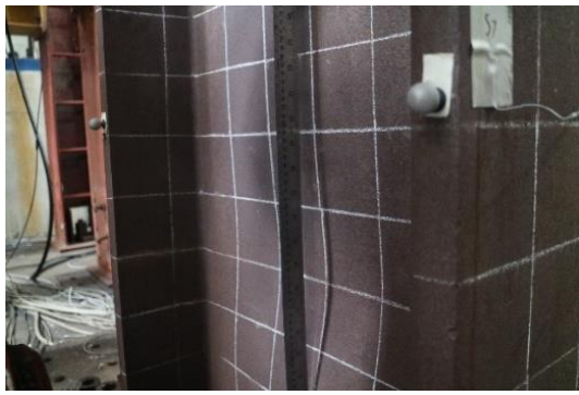
(a) 柱底腹板局部挫屈
