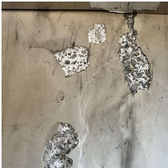
(c) 剝落 (攝於永福橋)
