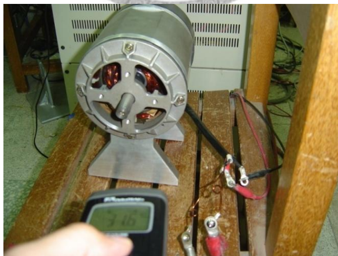
Fig. 6.32 The temperature measurement of the field winding
