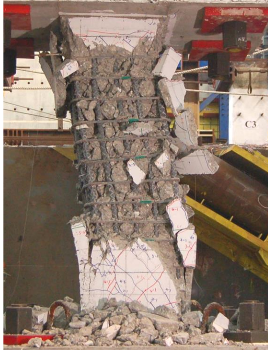
Figure 3-13. Specimen 3DL crack pattern before collapse (8%) (Weng 2007)
