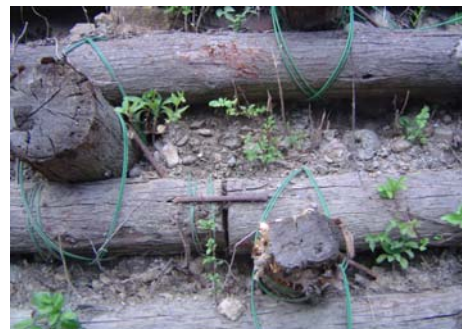
圖 9. 增加工程穩定性的螞蝗釘及鐵絲 Fig.9 The connection of retaining wall by leech staple and wire to increasing structure stability
