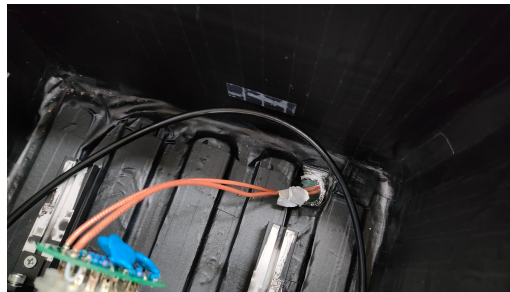
(c) The drilled hole to let cable pass through the black box.
