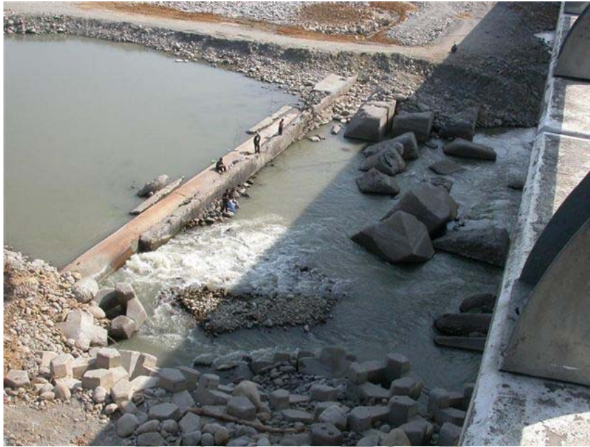
Figure 1.2 View of the exposed water main during low flow prior to the bridge failure. (photo courtesy of Zoe Lin, TBS)
