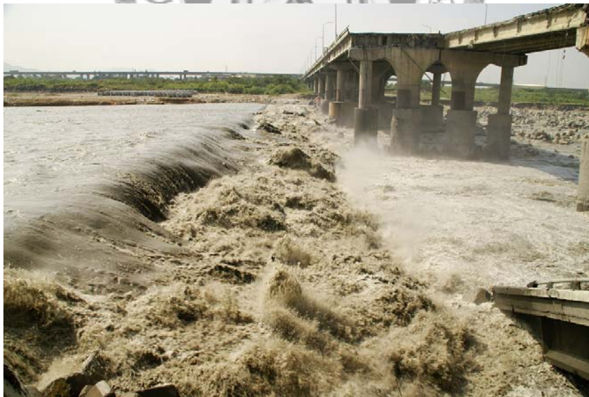
Figure 1.3 Failure of Hou-Feng Bridge connecting Houli and Fengyuan in Taichung due to Typhoon Sinlaku in October 2008. This view of the failed bridge a few days after failure. (photo by H.Capart)
