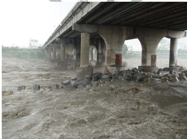
Figure 2.4 Local scour around four bridge piles.
