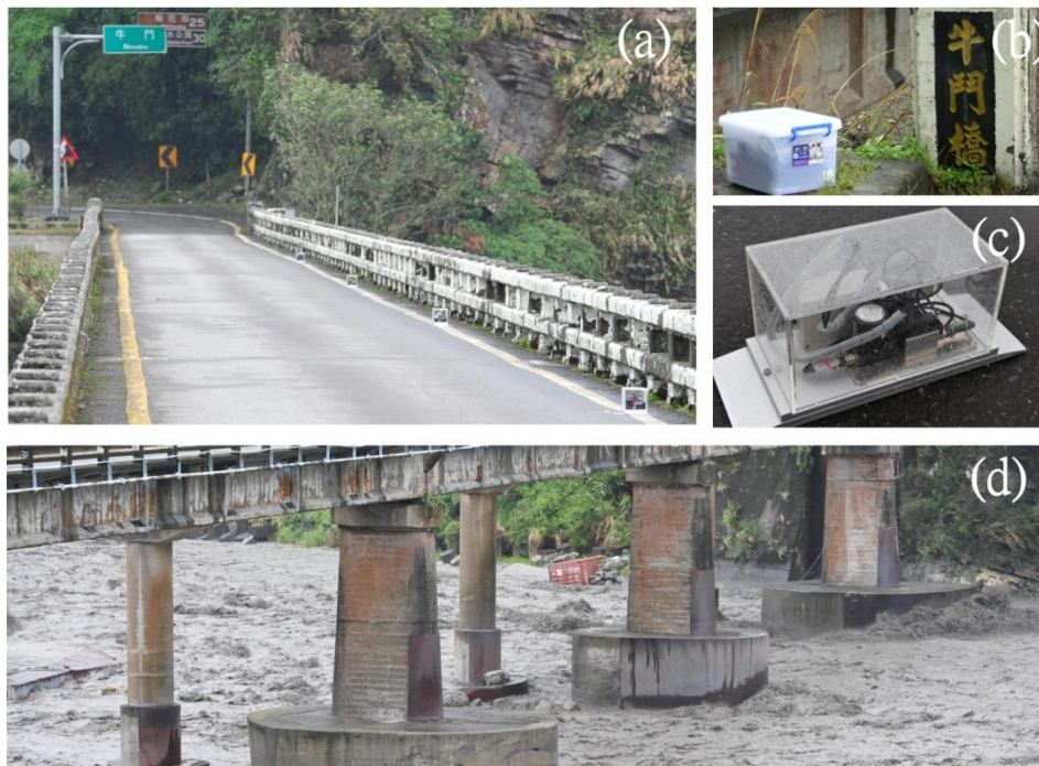
Figure 3.26: The photo of Smart Sensing System on Niudou Bridge
