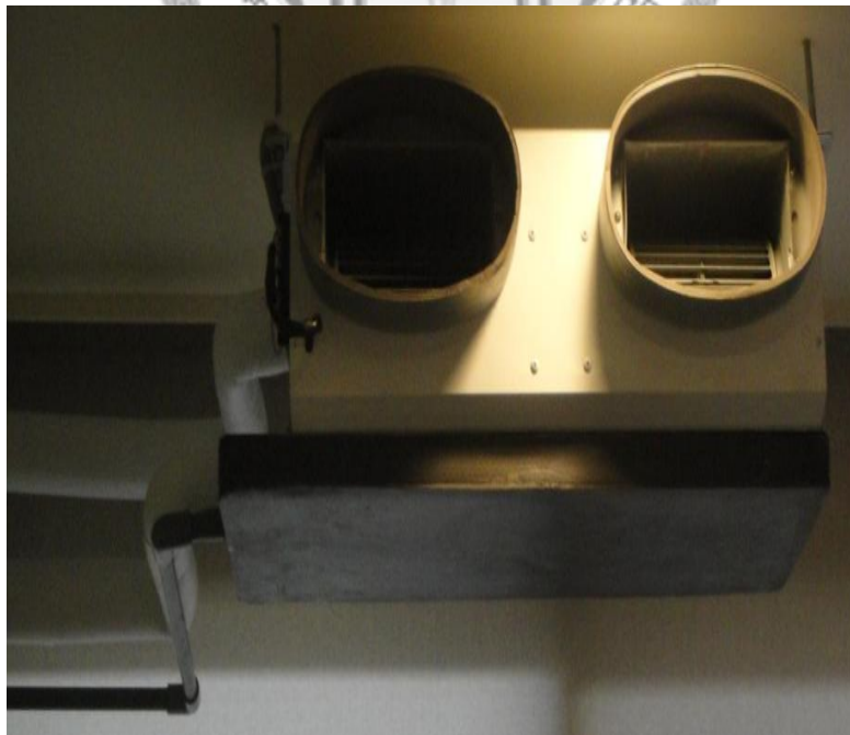
Modified Air-conditioner for the SEMD
