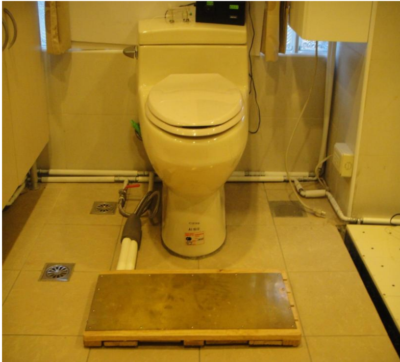
Floor Heating System
